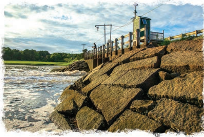
The Chequessett Neck Road dike at Herring River. Dikes, including this one, can block tidal flow between the ocean on one side and a marsh on the other. As part of the Herring River Restoration Project, conservation organizations and local stakeholders are working to remove the dike to restore tidal flow and stem the release of methane back into the atmosphere.
